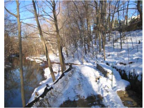
Snow blankets restoration work recently begun on the Bronx River path north of Hitchcock Pond in Scarsdale
